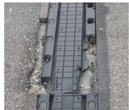
1 TENSACRETE expansion joint RE type 2 TENSACRETE expansion joint RE-LS type 3 Damaged bituminous expansion joint 4 Damaged mat expansion joint
