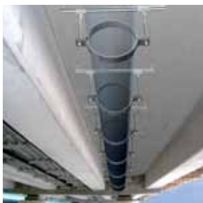
Water Pipeline and Other Supports
