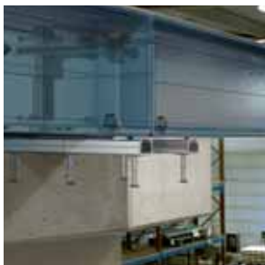
Overhead Crane Rails
