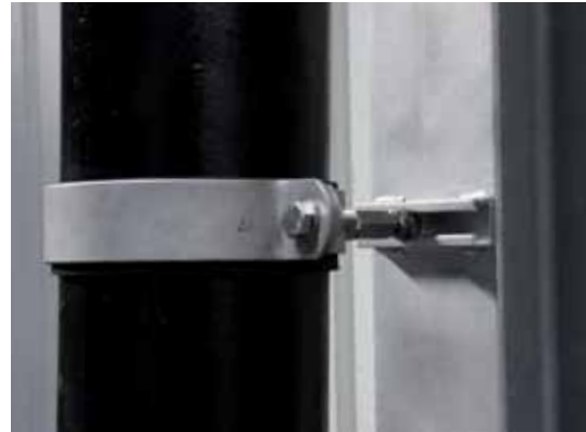
Welded Channel Supporting Water Pipe
