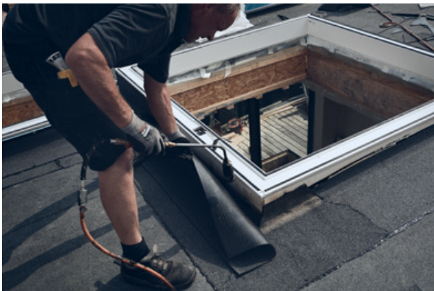
Securing the upstand and roofing material for watertightness without exposing the product to the flame.
